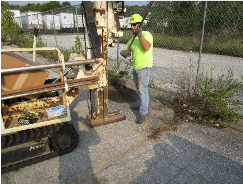
Photo 11: Installation of Boring PB-6 west of Leavenworth Animal Control Building; view to northwest.
