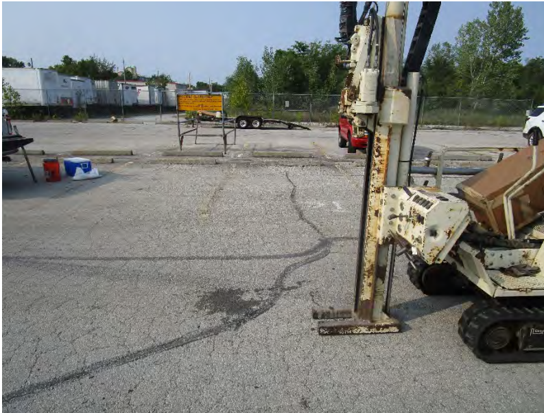
Photo 1: Installation of Boring PB-1A southwest of the Leavenworth Animal Control Building; view to north.
