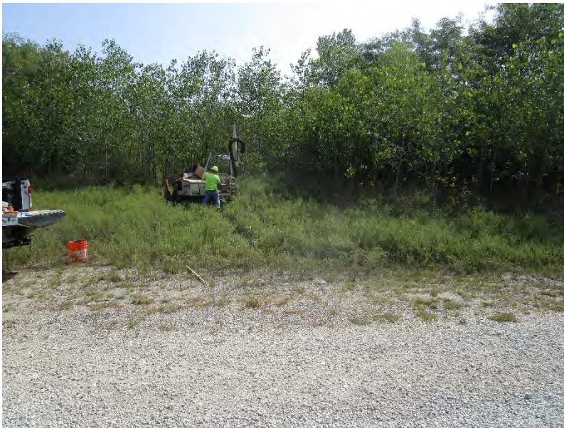
Photo 18: Installation of Boring PB-10 in northwest corner of the Subject Site; view to east.
