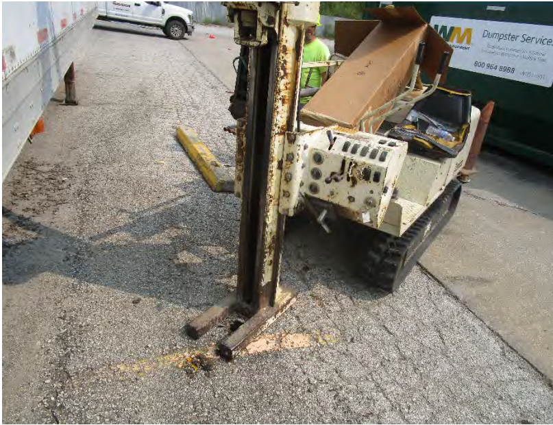
Photo 3: Installation of Boring PB-2 along south boundary of the Subject Site; view to east.
