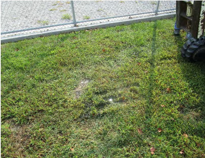
Photo 5: Installation of Boring PB-3 south of the Leavenworth Animal Control Building; view to southeast.
