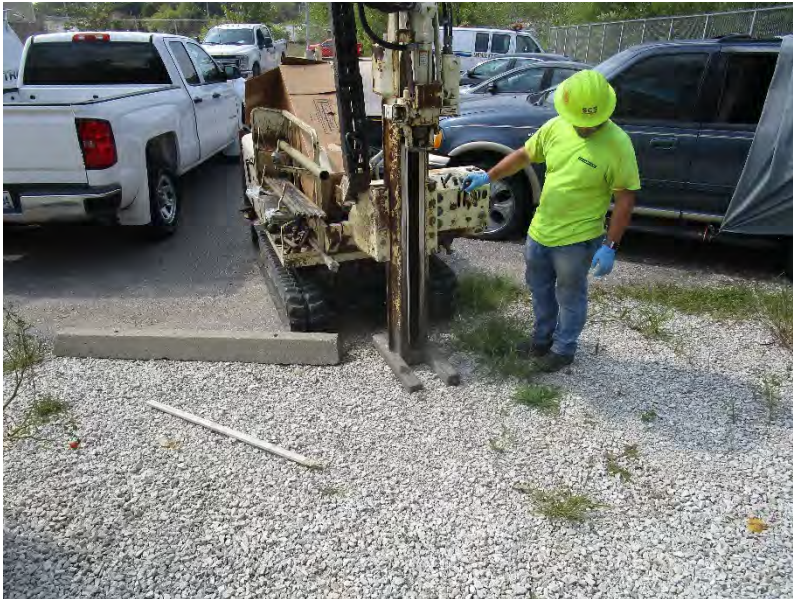
Photo 20: Installation of Boring PB-11 in northeast corner of the Subject Site; view to west.
