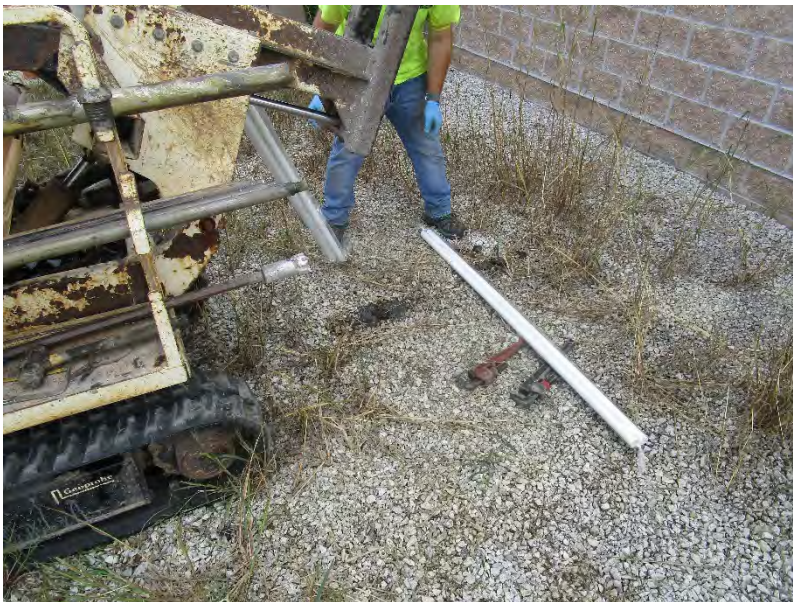
Photo 14: Installation of Boring PB-8 north of Leavenworth Animal Control Building; view to southeast.
