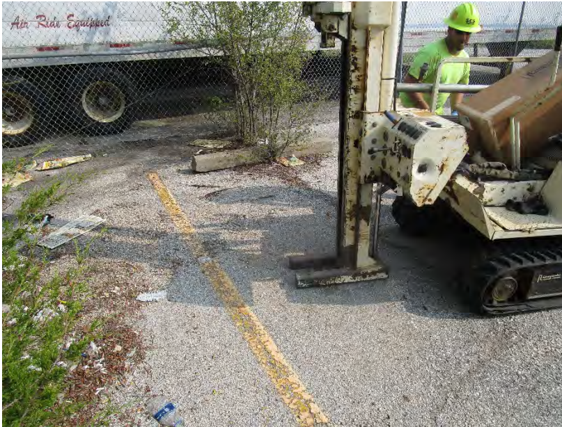
Photo 9: Installation of Boring PB-5 on west boundary of the Subject Site; view to north.
