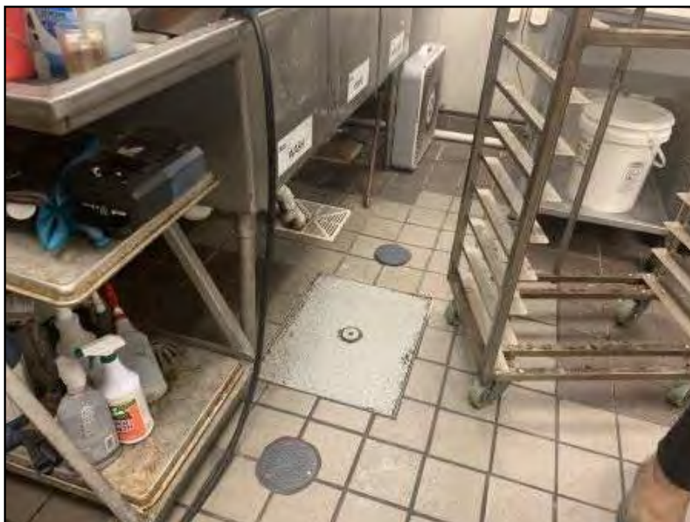
Northeast- View of a kitchen grease trap.
