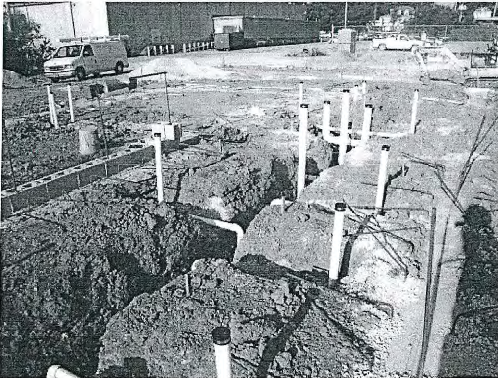
View of under slab plumbing in the west side of the Large Dog Adoption room, the restrooms, and the multi-purpose room
