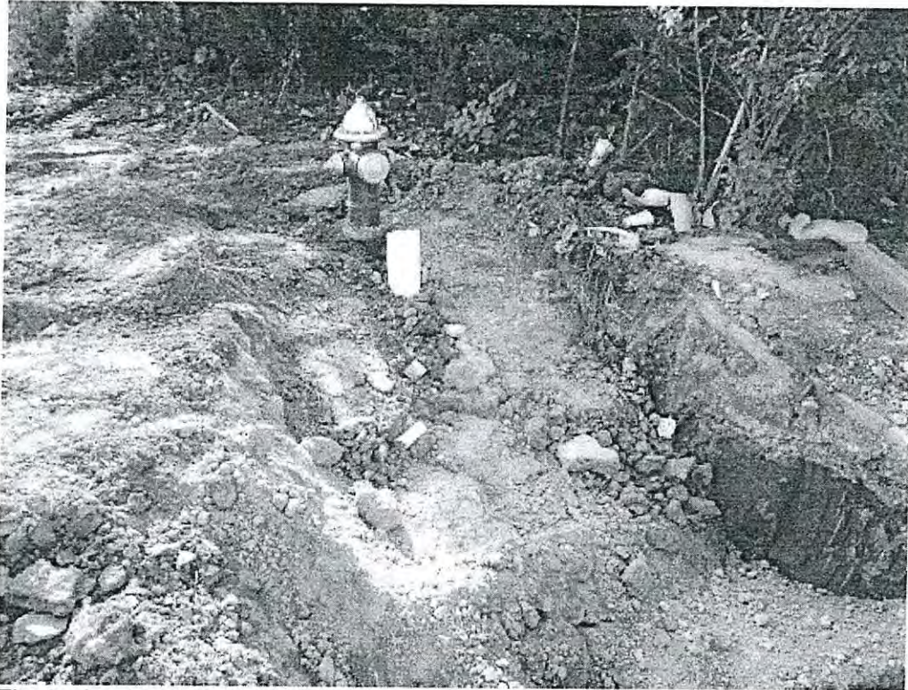
Fire hydrant installation with an incomplete valve box
