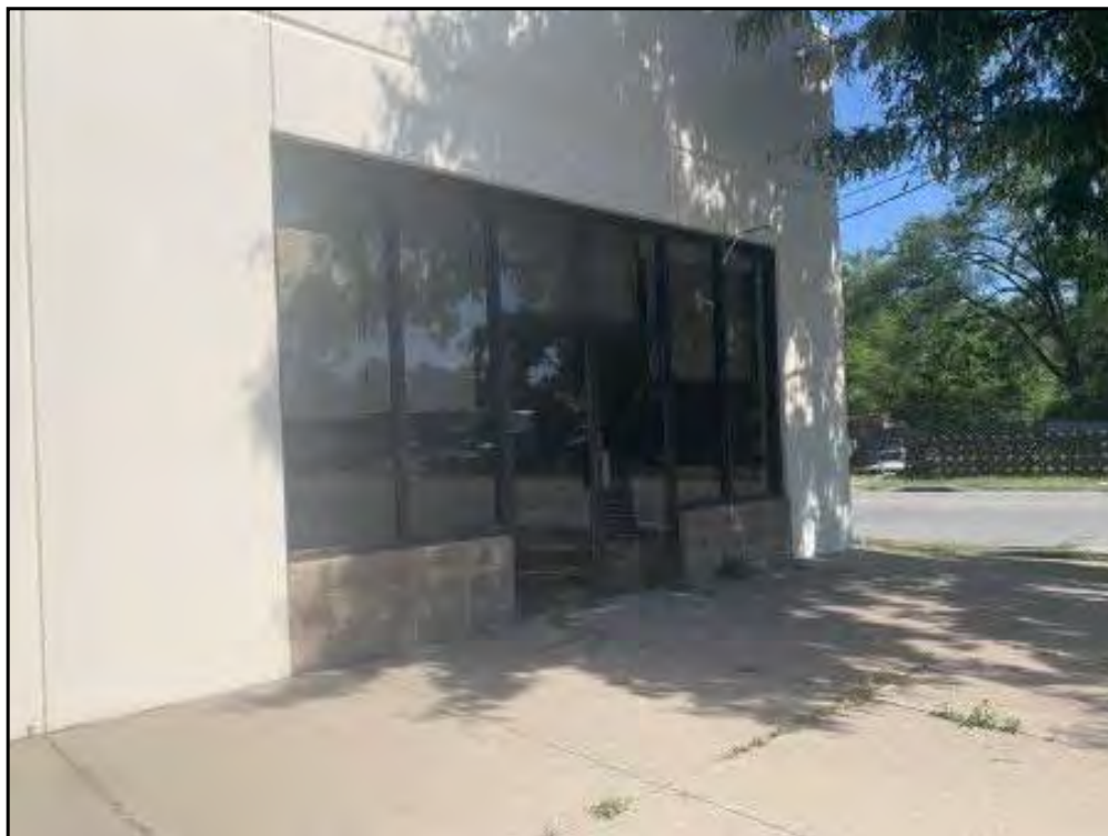
Southeast- View of the vacant tenant space on the southwest corner of the structure.
