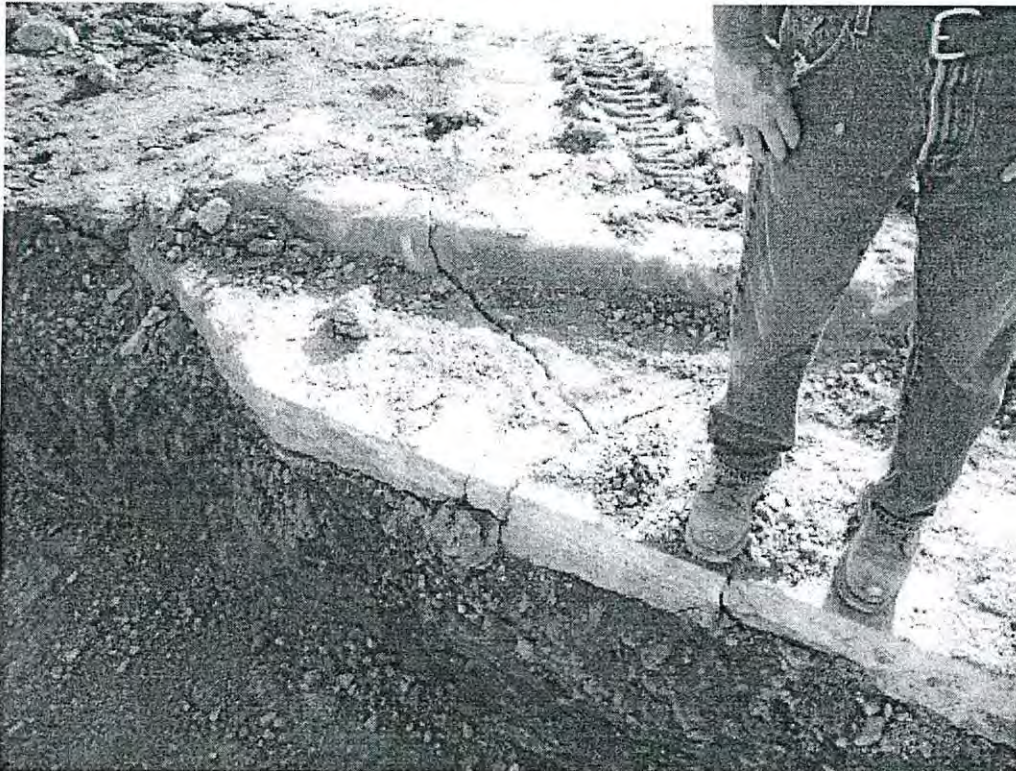
Damage to the concrete along the west side of the site, adjacent to the water line trench, damage presumably occurred during trenching, view to the east of the east side of the trench
