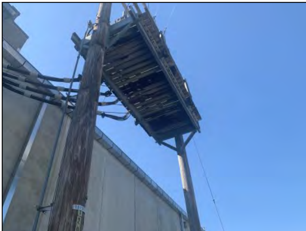
Northwest- View of the transformers located east of the structure. De minimis staining is visible on the platform beneath.
