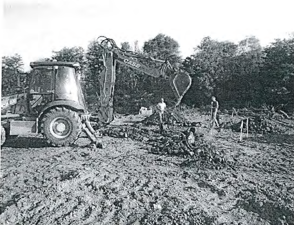
The excavator and rebar crew digging the trench for the trash enclosure footing
