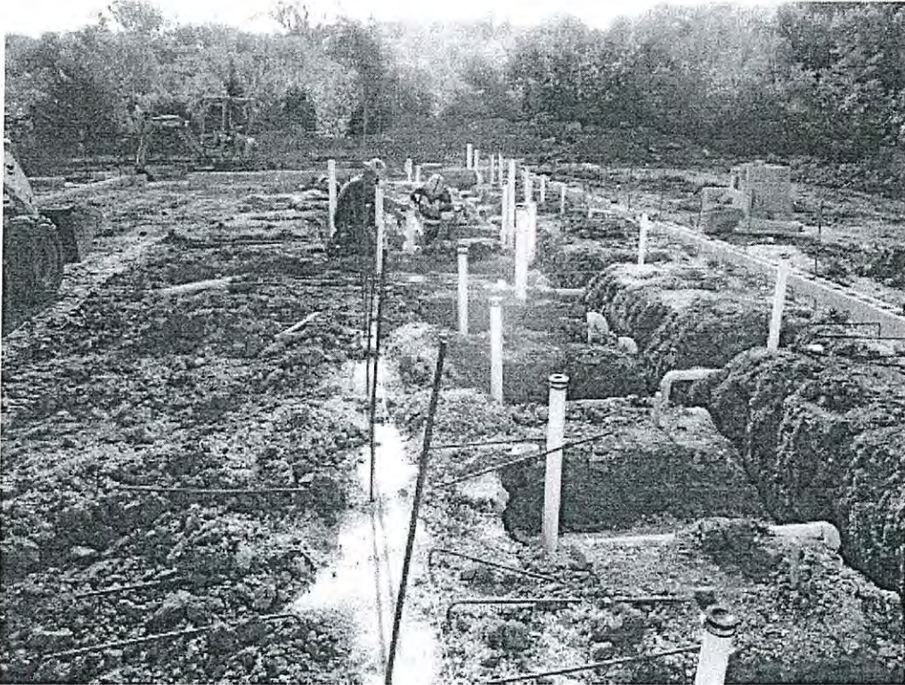
Plumbing along the south side of the building, view from center north wall of the Large Dog Adoption room
