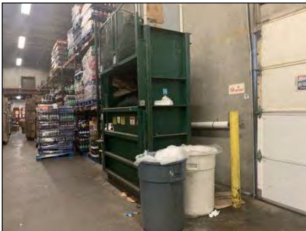
North- View of the hydraulic box compactor located in the back storage/stock area.
