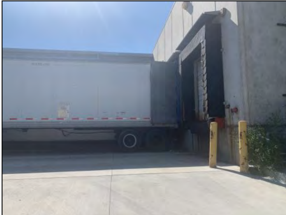
West- View of the loading docks on the southeast side of the structure.
