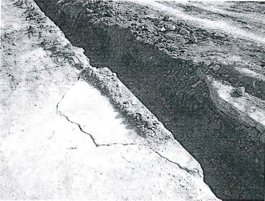
Damage to the concrete along the west side of the site, adjacent to the water line trench, damage presumably occurred during trenching, view to the north of the west side of the trench
