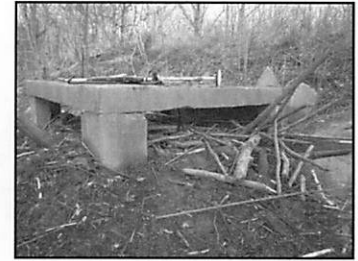
Outlet structure blocked with sediment and debris
