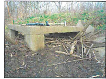
Outlet structure blocked with sediment and debris
