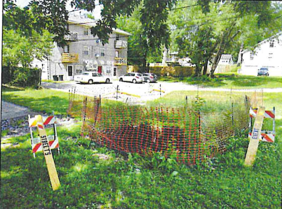
Many projects like this one at Second and Chestnut streets are in residential areas where sinkholes have shown up because of collapsed stormwater infrastructure. The City plans several stormwater repairs each year.
