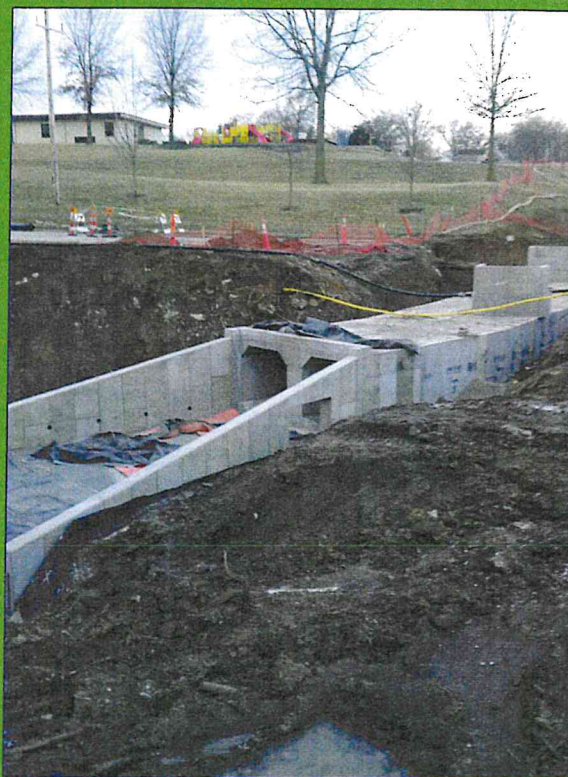
Work continued on the eastern portion of the City's major Thornton Street project near Anthony Elementary School in the winter of 2019-2020. These double reinforced concrete boxes to handle stormwater runoff. The next phase, set to begin in early summer, will close a portion of Thornton Avenue from 10th Avenue near Leavenworth High School heading east.
