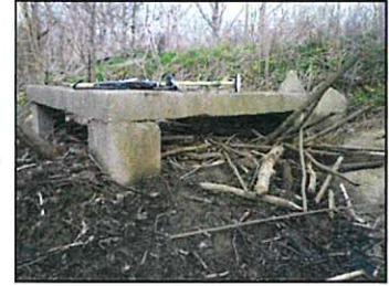
Outlet structure blocked with sediment and debris
