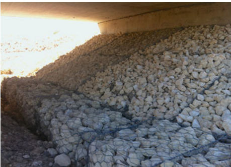
The City places riprap under bridges to protect the structure from erosion
