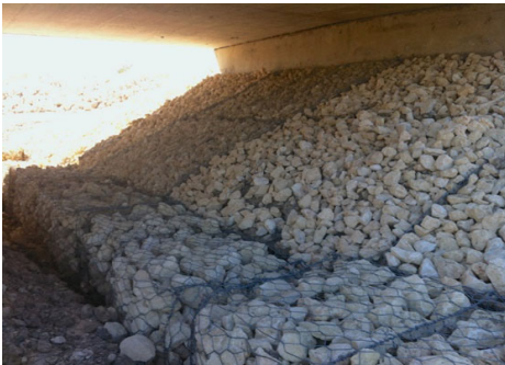
The City places riprap under bridges to protect the structure from erosion
