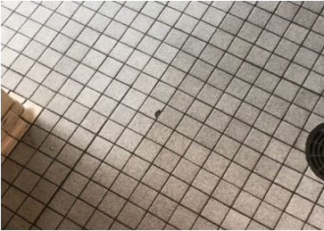
The current flooring is beginning to chip and could cause a safety hazard.
