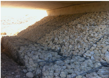
The City places riprap under bridges to protect the structure from erosion
