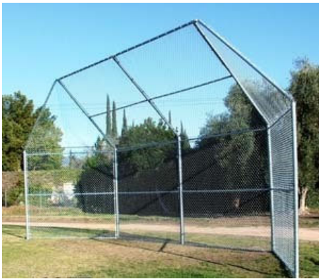
The current backstop is in need of replacement.
