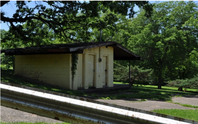
The current bathroom is beyond repair.
