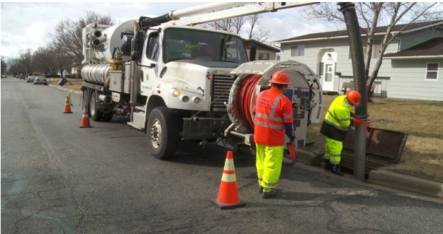
The vactor truck collects and transports sewage to the waste water treatment plant.
