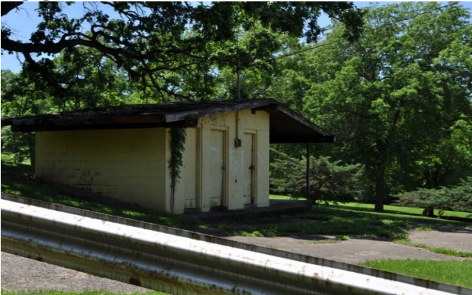
The current bathroom is beyond repair.
