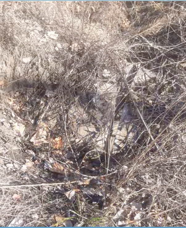
Figure 14. Separated 60-inch RCP end, Reach 3
