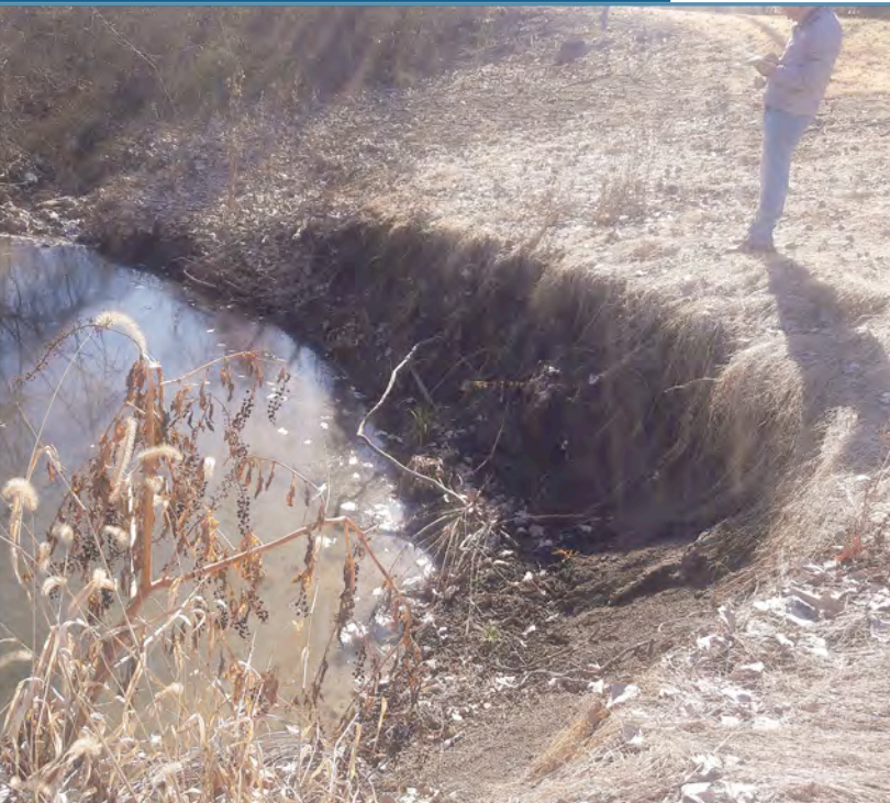
Figure 16. Scour at end of 10-inch RCP, Reach 3
