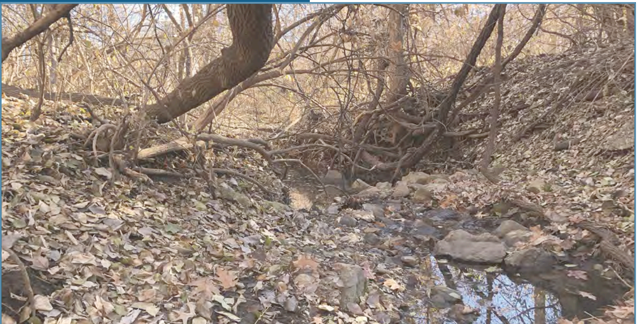
Figure 13. Displaced rock revetment, Reach 2
