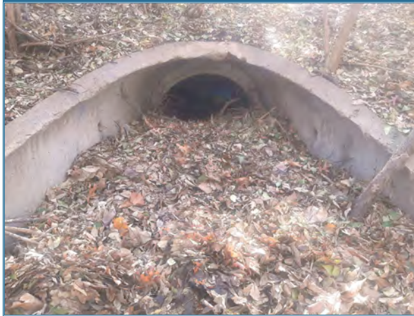
Figure 10. Debris filling pipe in Reach 1
