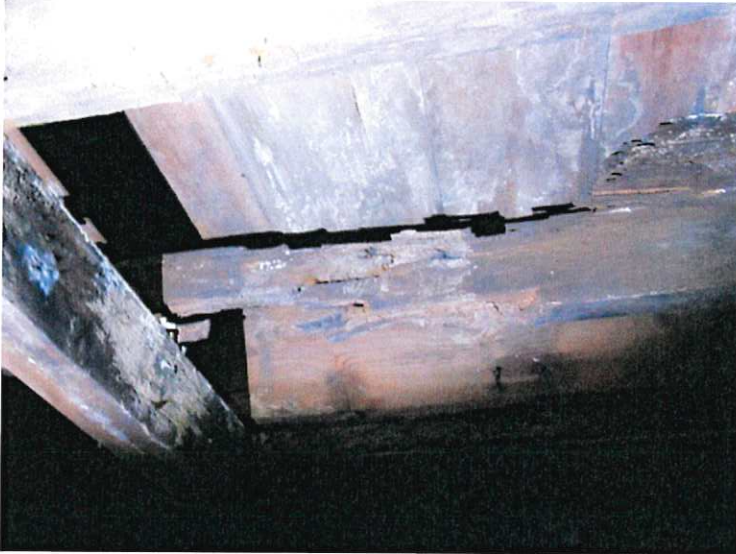
21. Close-up of a floor joist where the upper portions are missing due to extensive deterioration and rot problems.
