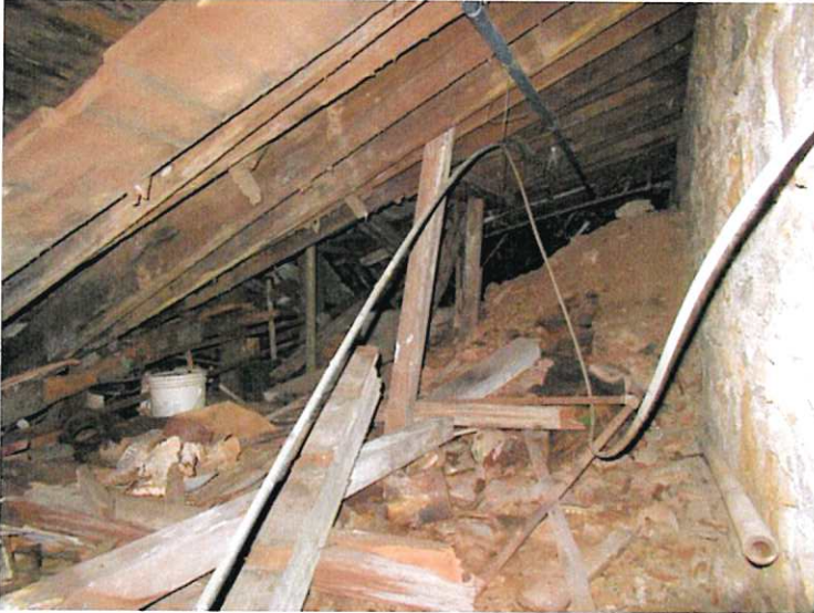
9. Looking north in the basement area at the collapsed framing.
