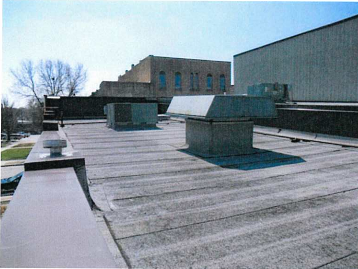
23. Looking south at the roofing on the east half of the building.
