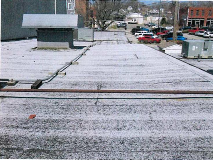
27. Low angle view of the roof showing the sag present in the roofing.
