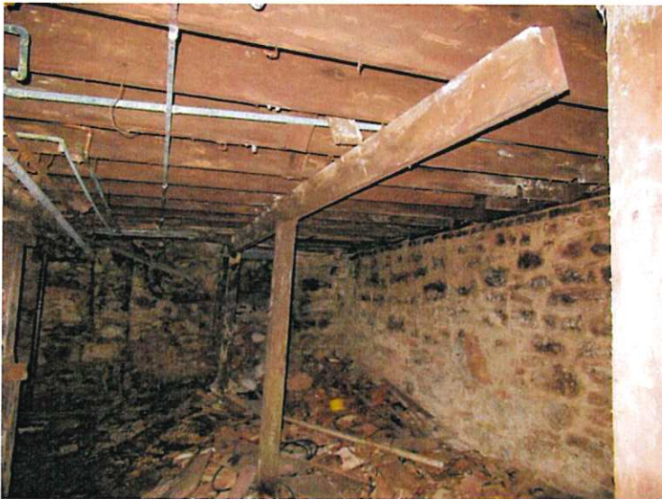
18. Another support post and column location that are rolling and tipping due to the extensive deterioration and rot problems.
