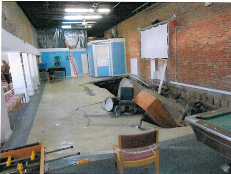
6. Looking south at the collapsed floor in the western half of the building.
