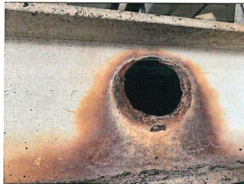
Holes Rusted Through Frame
