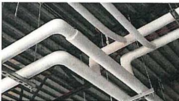
Condensate Piping System
