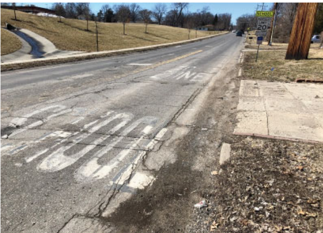
After listening to citizen feedback, the City Commission decided to invest in a street rebuild for Thornton Street.
