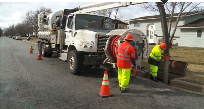
The vactor truck collects and transports sewage to the waste water treatment plant.
