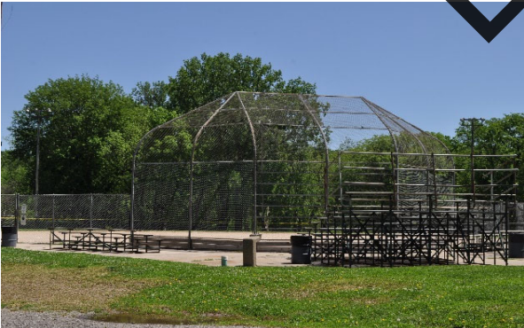
The fabric and some of the support post are in need of repair and replacement.
