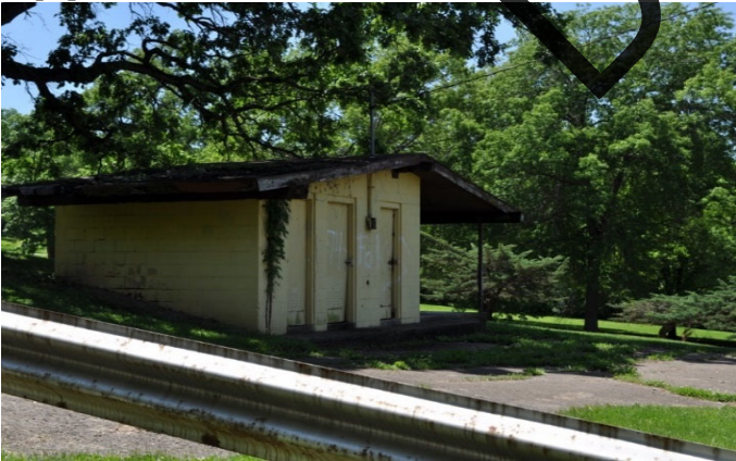
The current bathroom is beyond repair.
