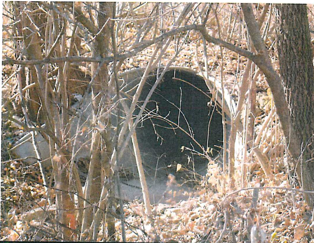
#8: The water then exits through this storm drain located between 1110 & 1028 Madison St.
