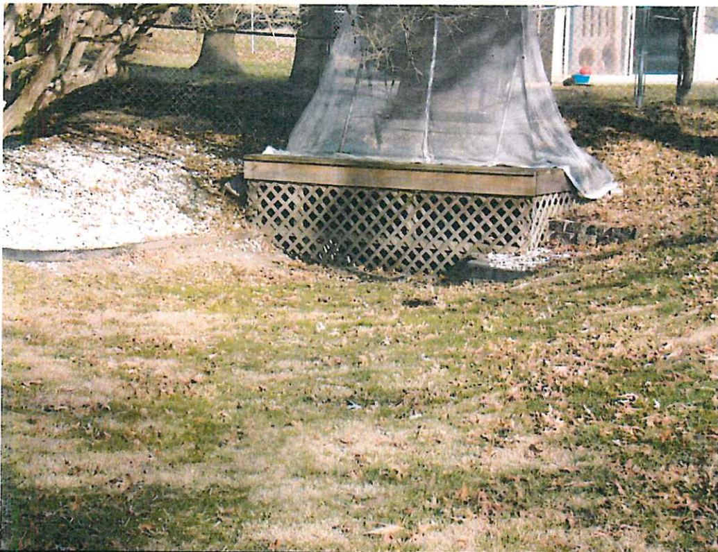
#4: The water from the woods and neighboring homes flows into this area of the back yard of 1106 South 14th Street and is diverted directly into this storm water run off tube.
