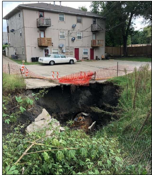
Figure 8: Sinkhole, September 2019, Looking Northeast
