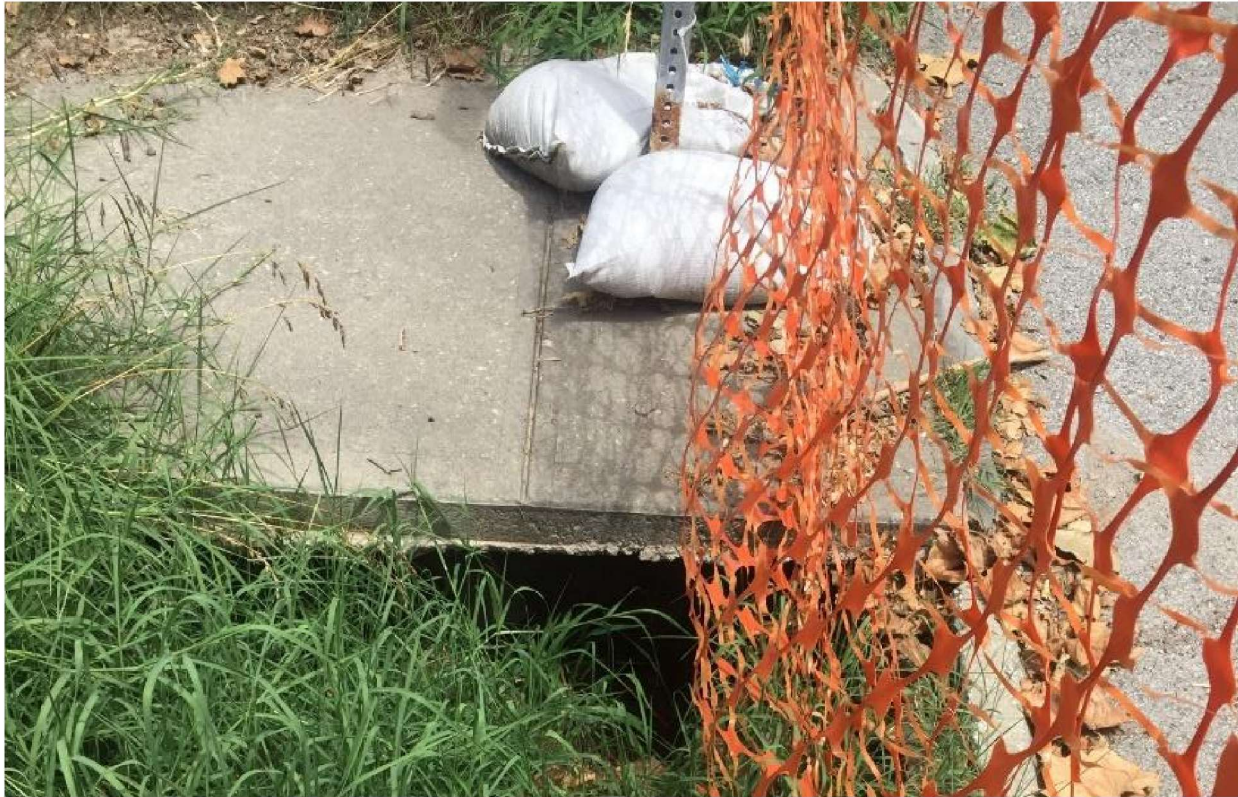
Figure 4: Sinkhole Under Sidewalk, Looking East
