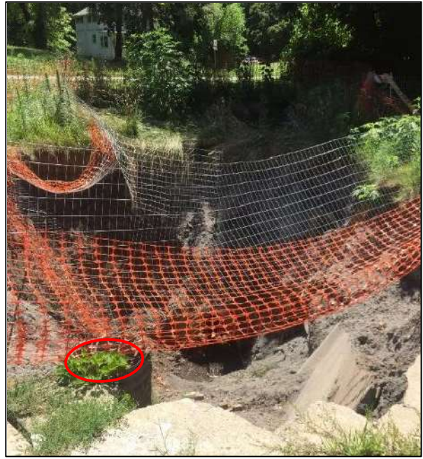
Figure 6: Sinkhole July 2019, Looking Southwest
