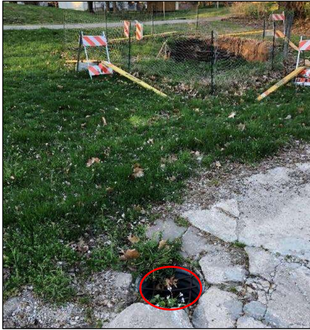
Figure 5: Sinkhole, April 2019, Looking Southwest
