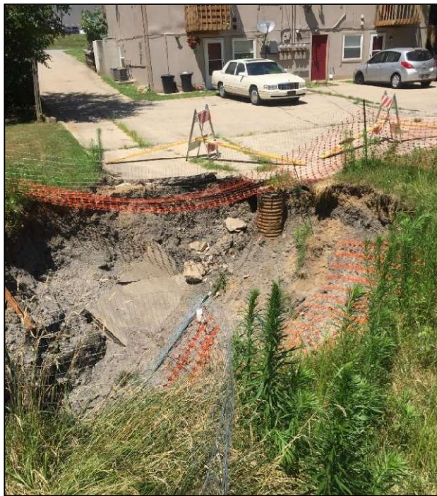
Figure 7: Sinkhole, July 2019, Looking Northeast
